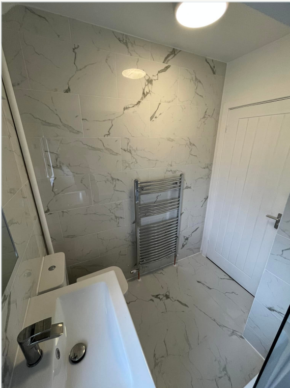
Wall panels and towel radiator
